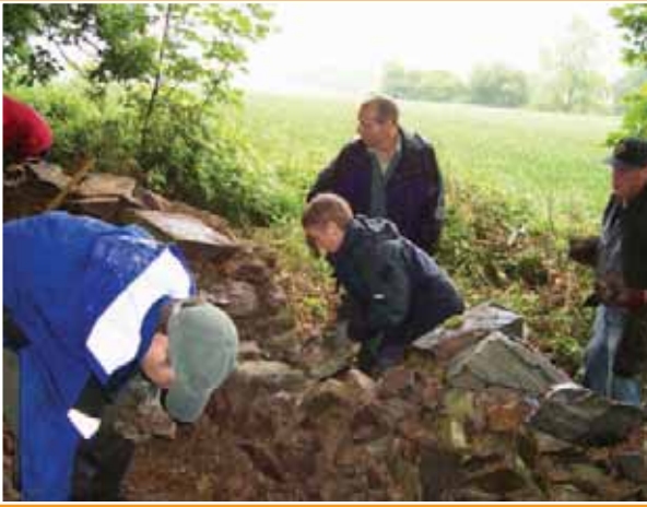
Grant Thornton spend a day in the pouring rain at the Outwoods doing drystone walling and fence building
